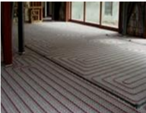
Radiant Floor Heating
