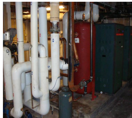
Commercial Boilers/Hot Water Heaters
