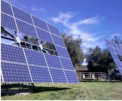
Ground-Mounted Solar Photovoltaic
