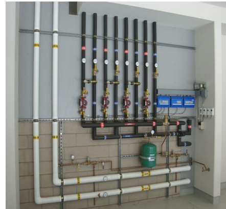
Mechanical Piping & Controls for Radiant Floor Heating
