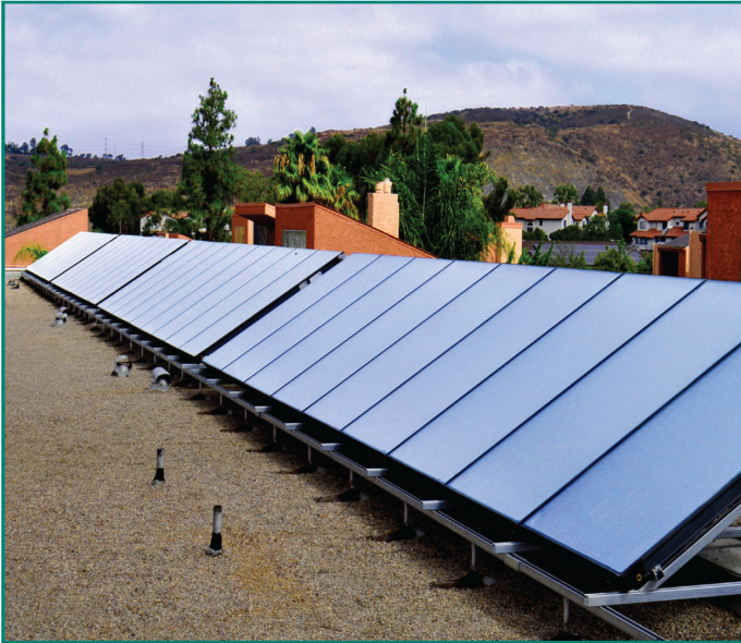
The largest of the three systems has 36 Buderus SKN 3.0 collectors, and a 1,200 gallon Haase Energy storage tank.
